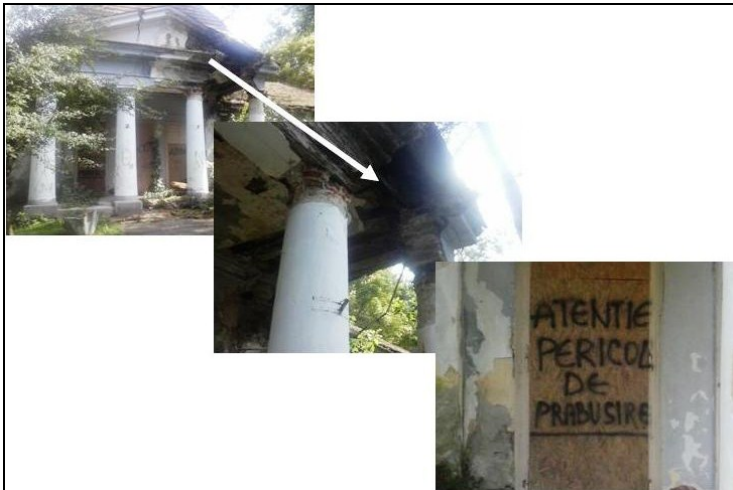
Figure 3. Ruined and abandoned building in the resort of Buziaș with high potential of risk for local community. A glance on the lower-right image meets the message: “Caution, danger of crash”
