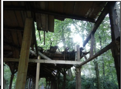
Figure 11. Collapsed roof above a park alley
