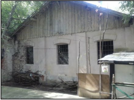
Figure 7. A derelict building, once included in the spa resort
