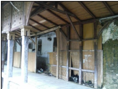
Figure 9. Damaged section of Buziaș touristic park
