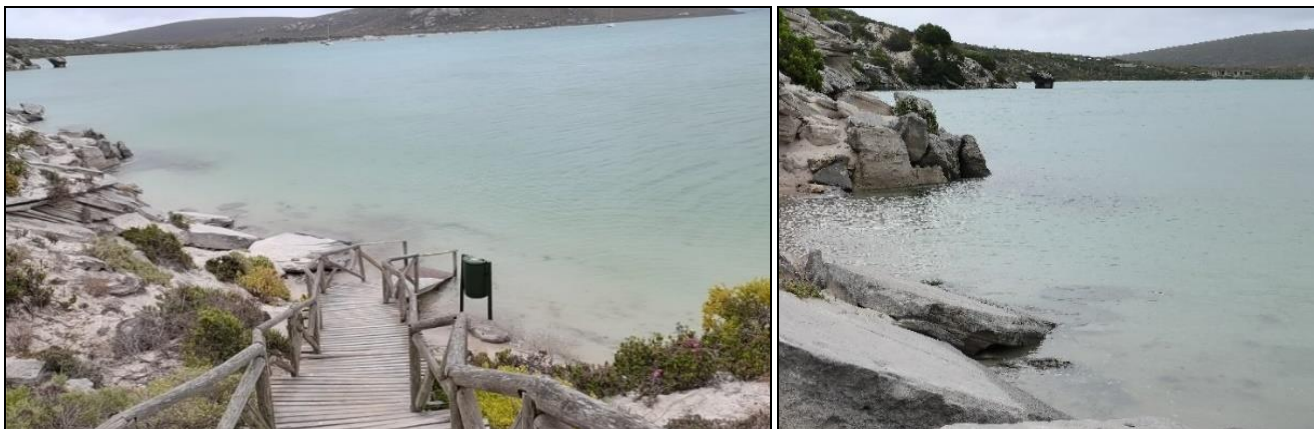
Figure 5. Inundated beach, collapsing walkways and large chunks of eroded earth at the West Coast National Park
