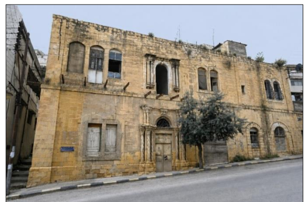
Figure 16. Falah Al-Hamad House (1890–1918): ornate Art Nouveau entrance portal and yellow limestone masonry, now deteriorated and awaiting restoration (Source: Authors)
